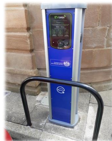
Electric Vehicle Charger
